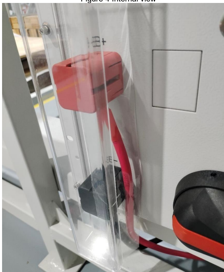
Figure 5 B+/B- terminal view
