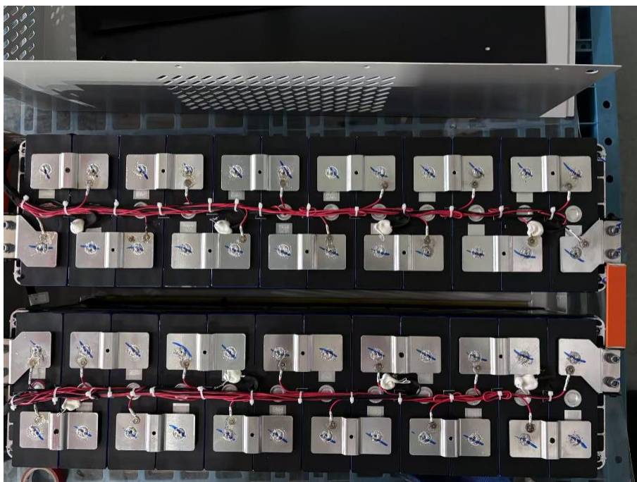
Figure 20 Internal view for battery module
