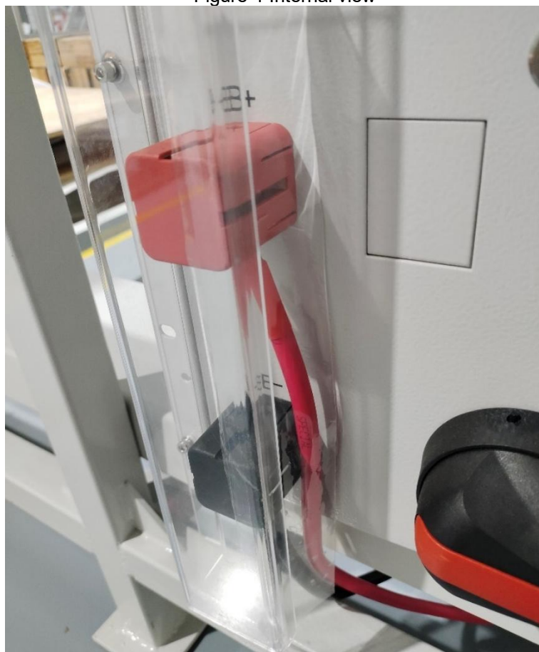
Figure 5 B+/B- terminal view
