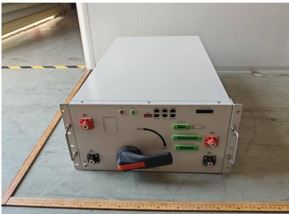
Figure 7 External view of high voltage control box
