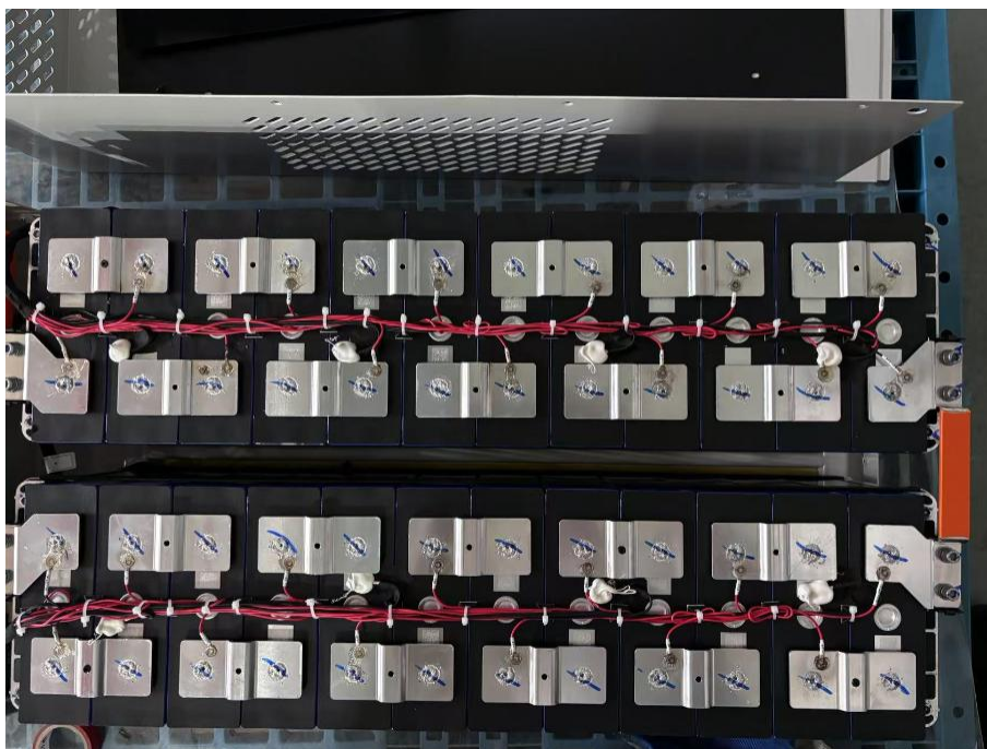
Figure 20 Internal view for battery module
